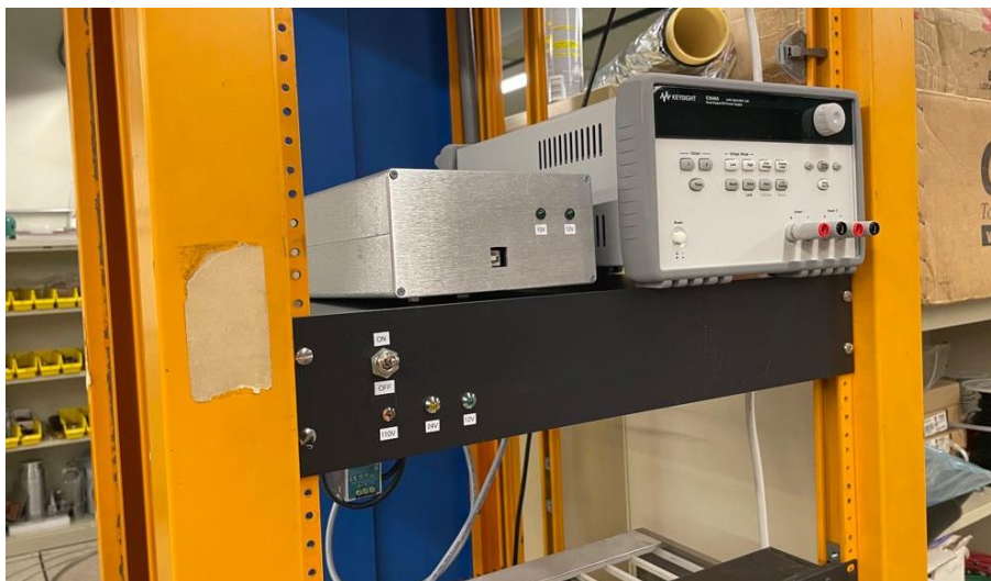
Figure 5 : Placement of the control box on the slow control rack
