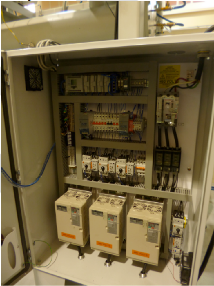
Figure 11: Electrical control panel for roots power supply
