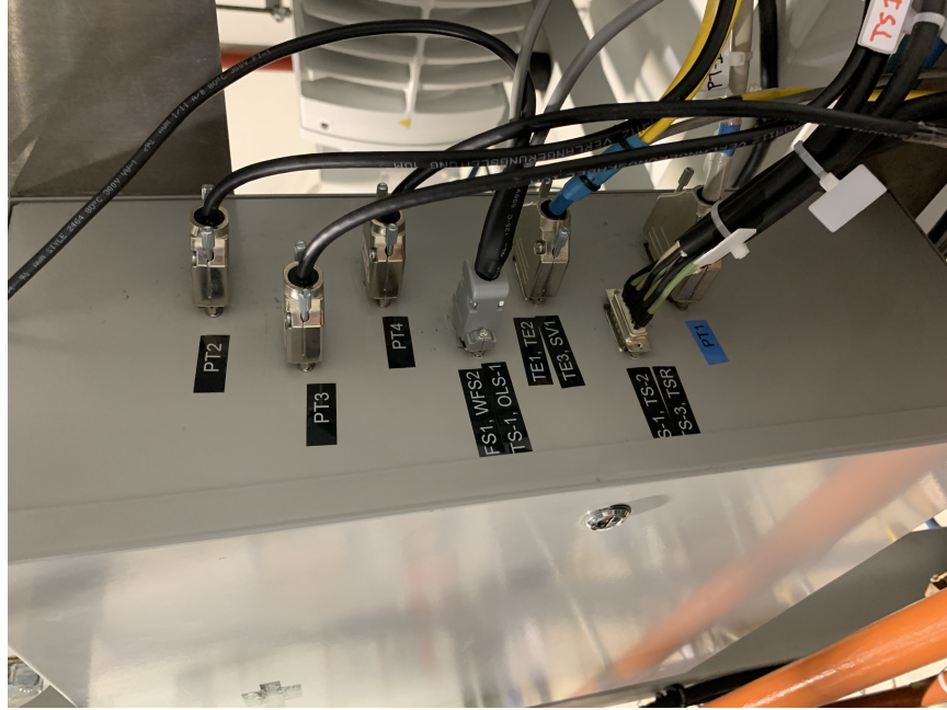
Figure 7: 24 VDC feedthrough panel
