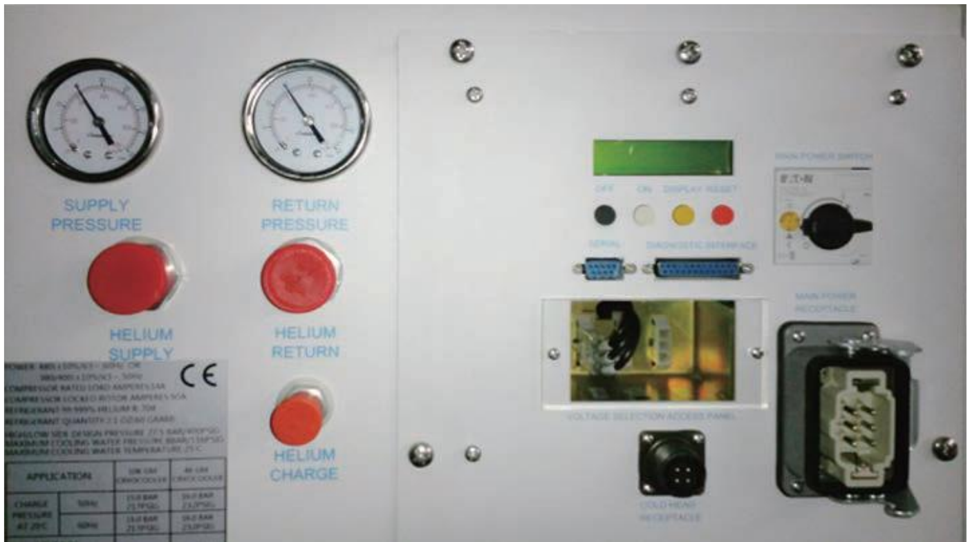
Figure 5 Electrical Control Panel
